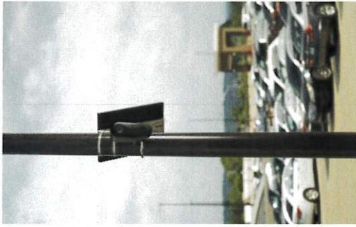
Solar & Existing Pole
